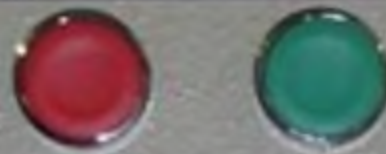
SHAFT GEN. CIRCUIT BREAKER OUT/RESET IN
